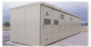
High-voltage power receiving
